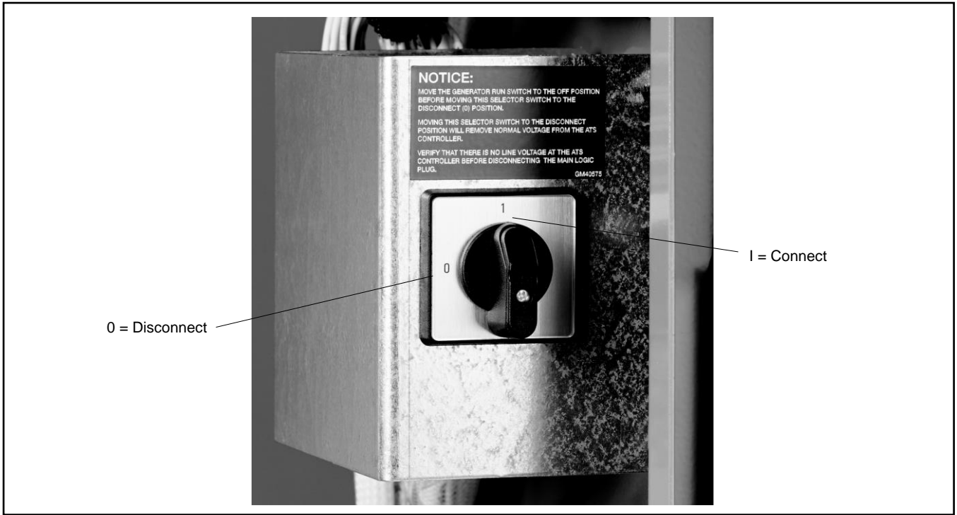
Figure 69 Controller Disconnect Switch
