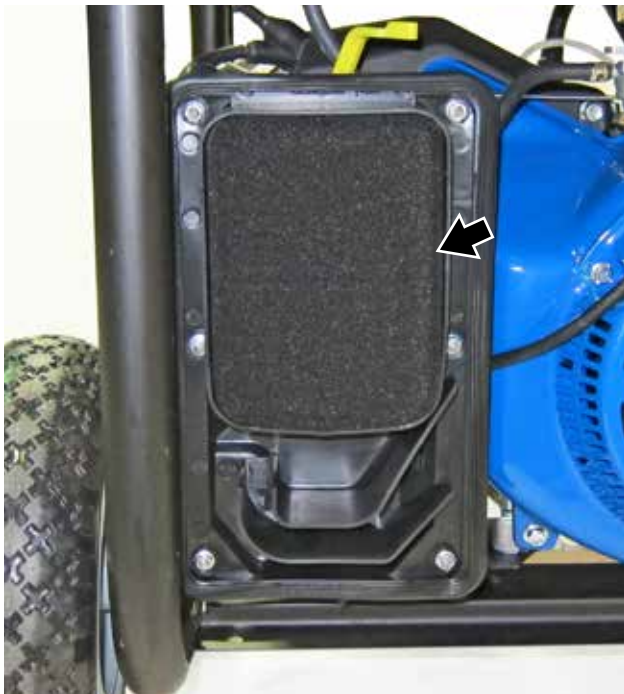
Figure 31 – Removing Coarse Outside Air Filter
