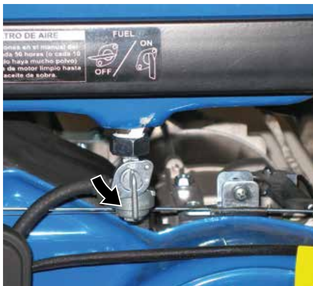
Figure 22 – Fuel Shutoff Valve in the ON Position
